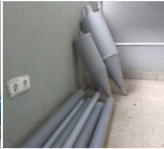
(b) pipe line and cyclone separator
