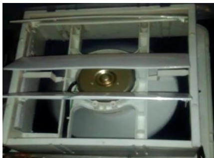
Figure 11 Humidity sensor and fan in operation
