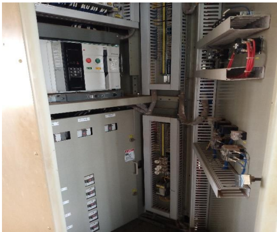
Power distribution panel
