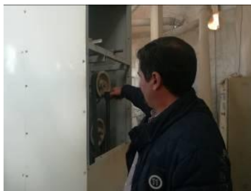
Figure 4 Using an optical tachometer (model Pantec DTM 30) to determine the rotational speed of the machine axis
