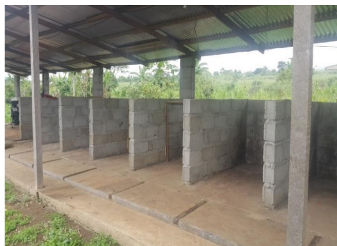
Figure 1 Roofed composting facility showing empty composting chambers, each with three walls and one open side
