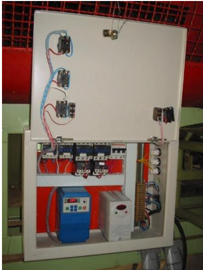
Figure 5 Internal parts of the electrical system and speed control of electric motors
