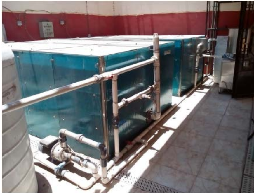
Figure 2 The portable assembly biogas unit under investigation
