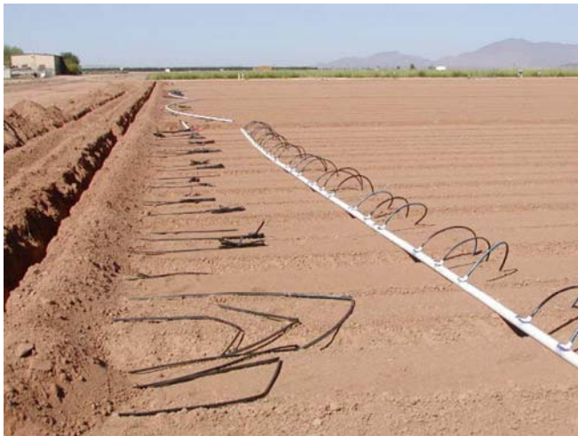
Figure 2 Drip system establishment and installation automated controller surface and subsurface drip irrigation systems in new field
