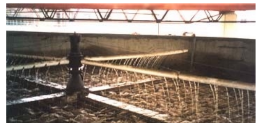
Fig 17. Pig farms wastewater treatment
