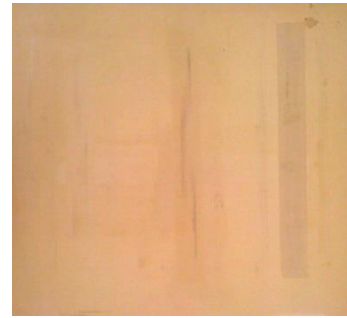
Figure 5 Floor panel in resin A after the test. The mark of red wine is evident
