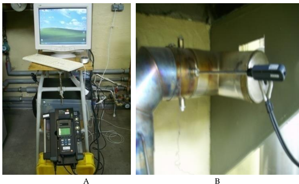
Figure 4 A - Emissions analyzer TESTO 350 XL connected to the computer, B - Sampling probe emission of analyzer connected to the smoke flue
