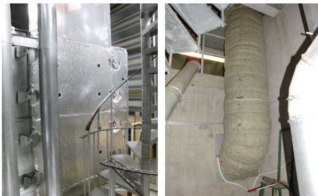
Figure 3 Heat insulation of the drying silo and the incoming drying air pipe
