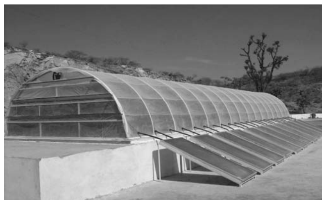
Figure 1 Solar tunnel dryer at M/s Miraj Products Pvt. Ltd., Nathdawara
