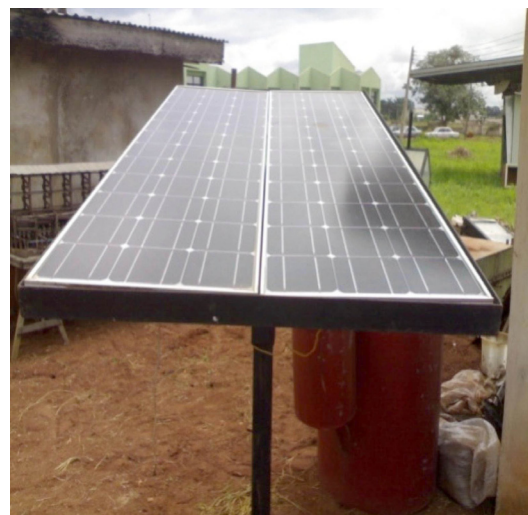
Figure 3 Picture of the Solar PV modules
