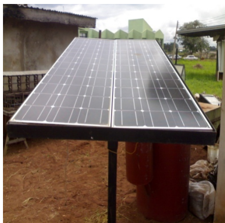
Figure 3 Picture of the Solar PV modules.
