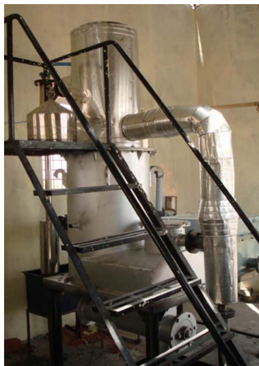
Figure1 10 kW biomass gasifier installed at energy park UIT-RGTU Bhopal
