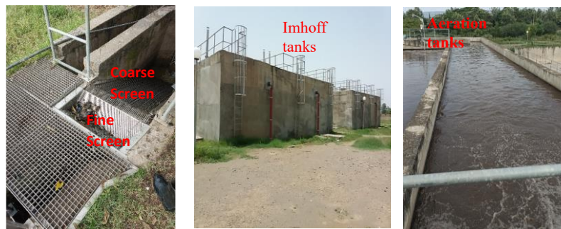
Figure 1 ASTU Wastewater Treatment Plant
