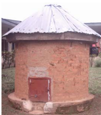
Figure 7: Completed silo showing the manhole to which the discharge chute is attached
